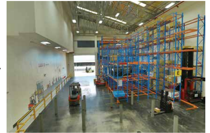
The various racking systems for live demonstrations at the new Technical Training Centre
